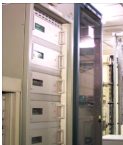
Figure 5 – Inverness Equipment Room
