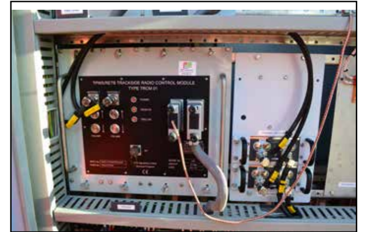
Figure 13 – Trackside Radio Control Module (TRCM)
